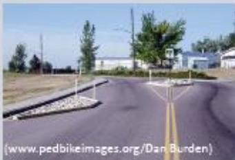
(www.pedbikemages.org/Dan Burden) Chicaines are a series of raised curb extensions on alternating sides of a street forming an S-shaped travel way, reducing vehicle speeds.
