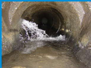
Infiltration from cracks in sewer line
