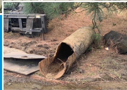
Over 50 year old corrugated pipe failure
