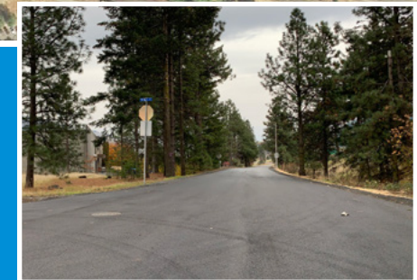
Looking east down Riverside Drive from North 8th Street after Phase 1 construction
